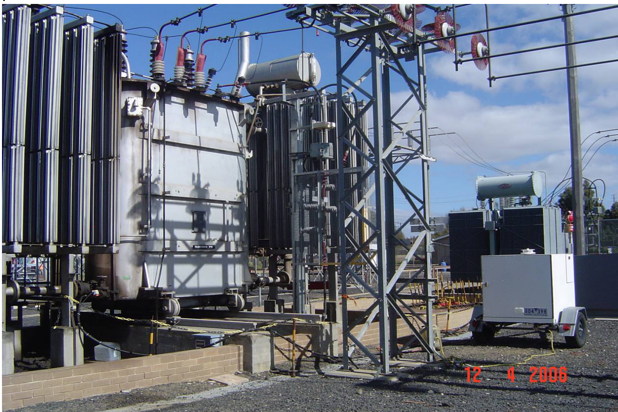
Trojan 1000 connected to the transformer
